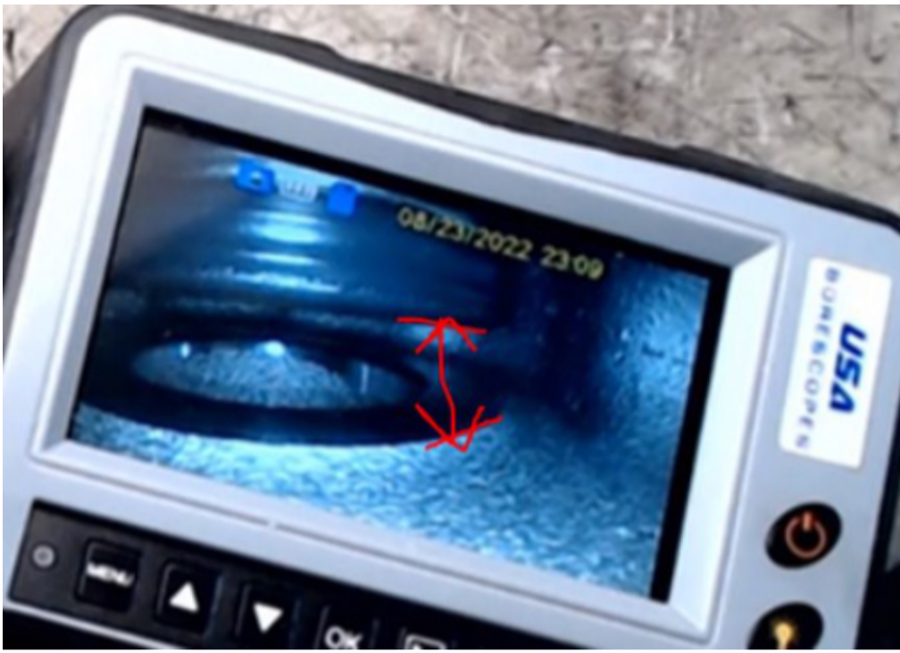
Picture below shows Charge Air Bypass Valve in stuck open position (plunger fully retracted)
