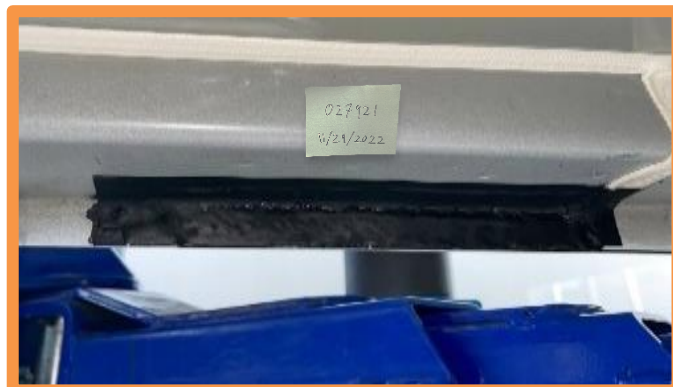
Example of acceptable STUI photo
