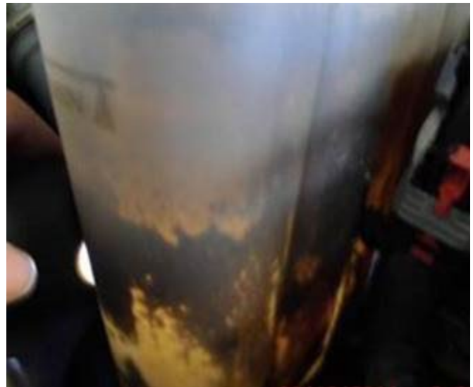
Figure 12. Discolored coolant expansion tank.
