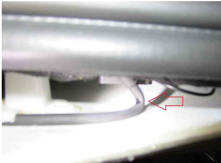
Sharp bend above headliner restricting washer fluid flow
