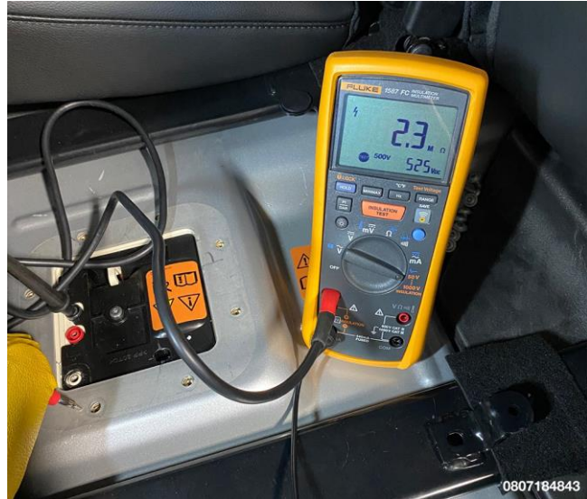
Figure 29 – Measure and Record Isolation Resistance Between HV Negative Test Point and Chassis Ground
