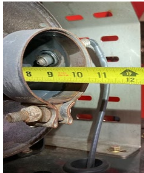
INCORRECT Catalyst Depth
