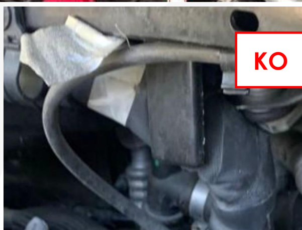
Example of incorrect routing BEHIND the plate
