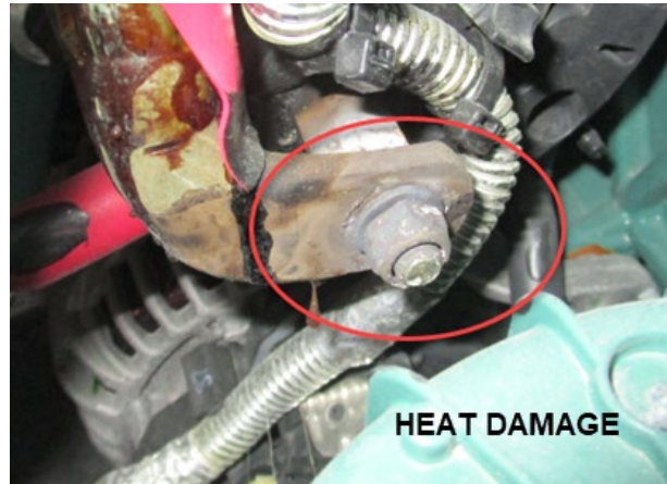
Figure 4: Example of discoloration caused by heat damage
