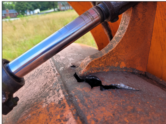
Crack with Over \frac{1}{8} " Material Separation
