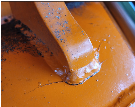
Crack with \frac{1}{8} " Separation or Less
