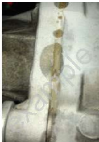
Figure 1. Bevel box case seam leak location.
