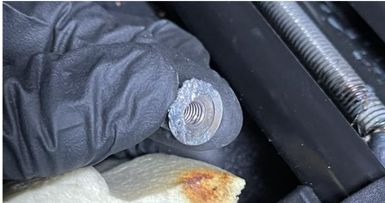
Ground Stud Nut Damaged By Arcing
