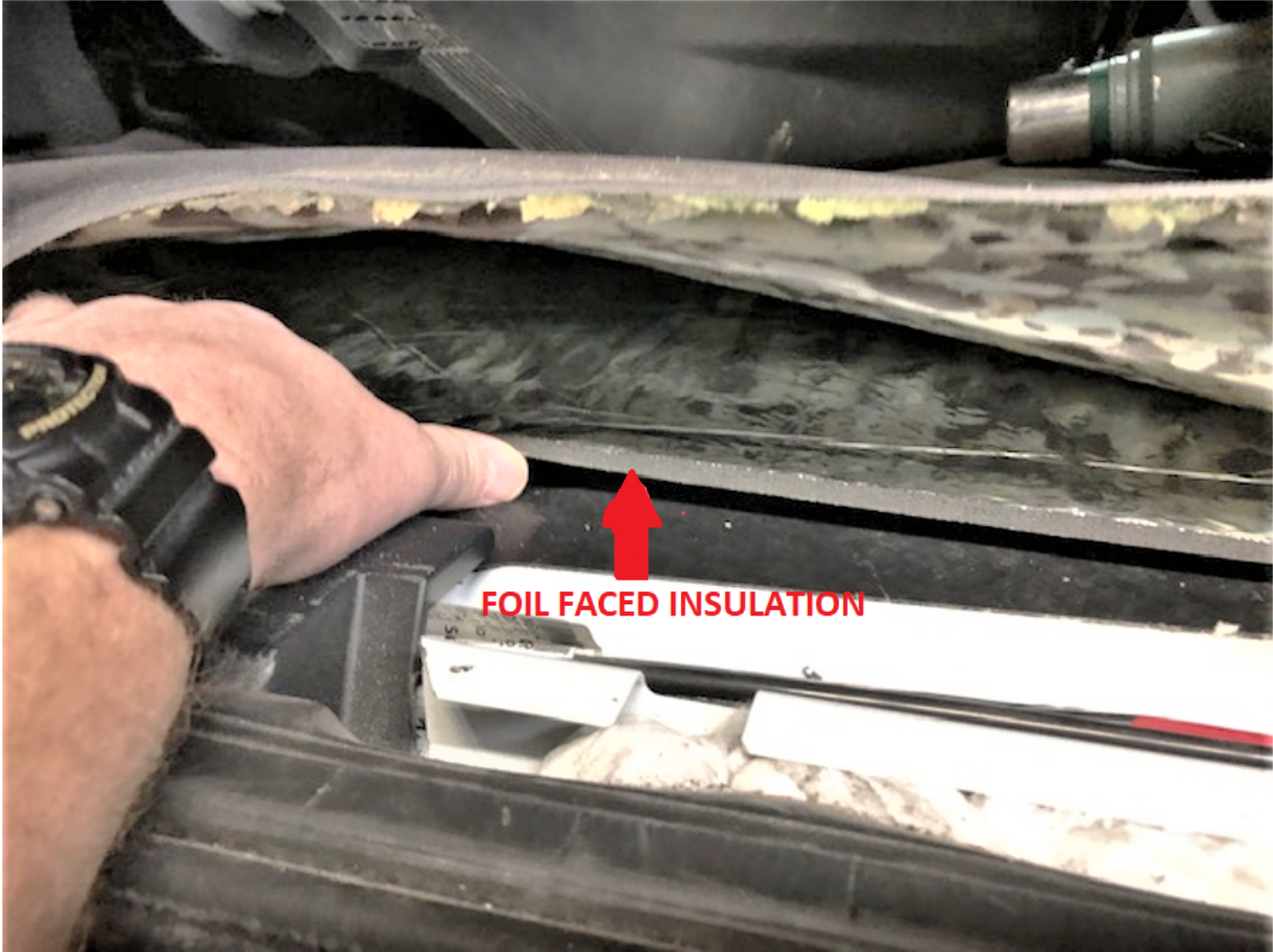
Figure 4 Added insulation (foil faced) to be removed as documented in figure 2 or figure 3 depending on the drive position.
