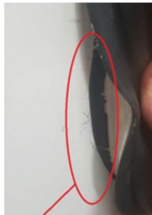
FIGURE 10 POOR BUTYL ADHESION TO WALL
