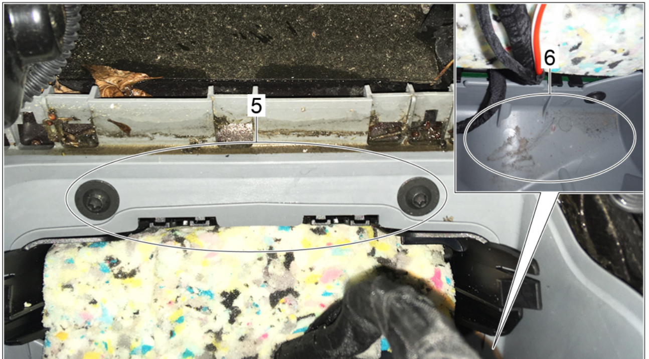
Water leak in fuse box
