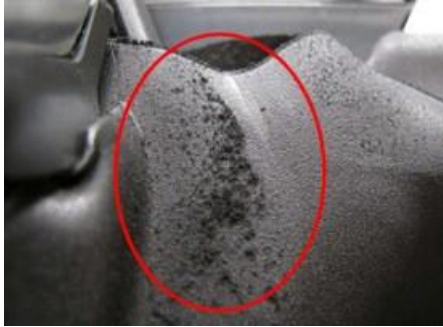
Figure 4 (Door seal worn)
