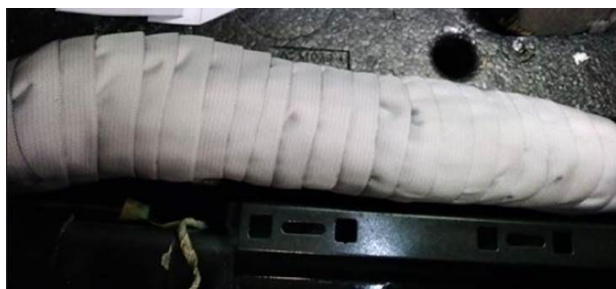
Figure 11: Gray textile tape covering the already wrapped main wiring harness.
