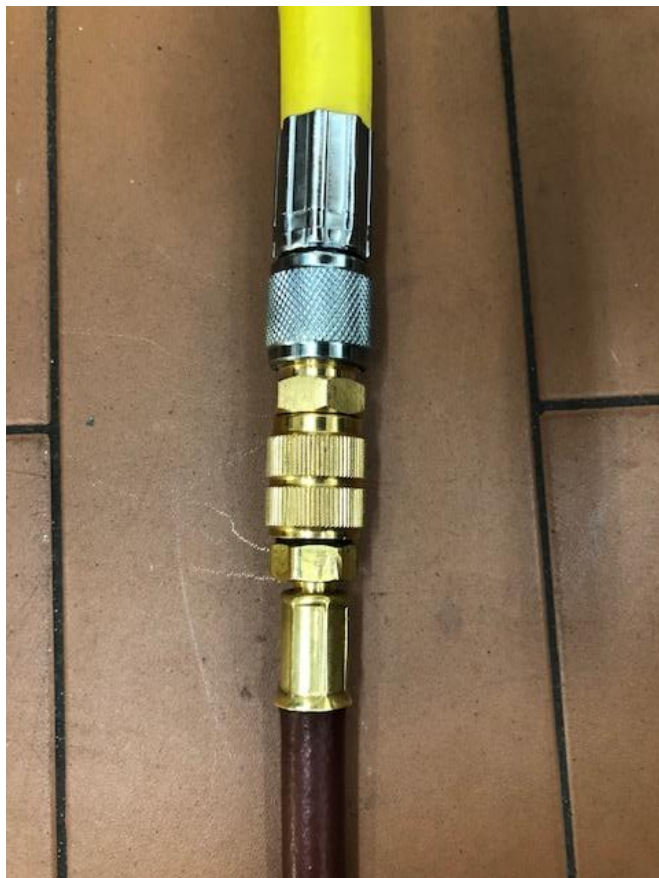
18. Y1234a high side adapter installed in place of the quick disconnect
