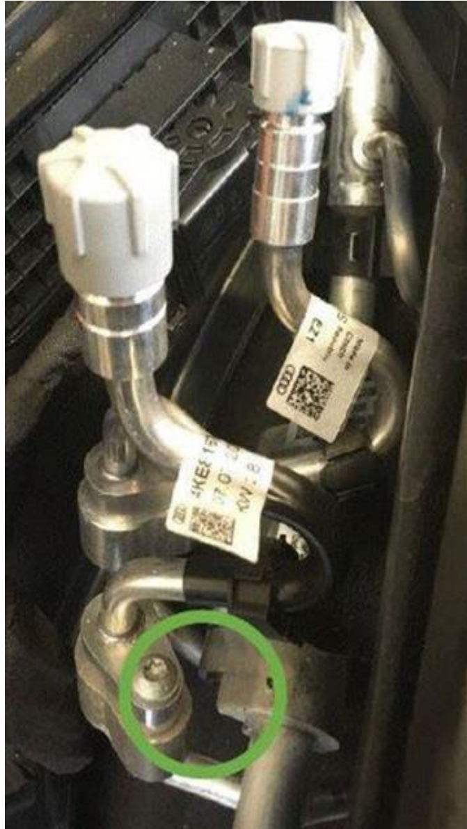
Figure 6. Refrigerant lines retained in a separated position.
