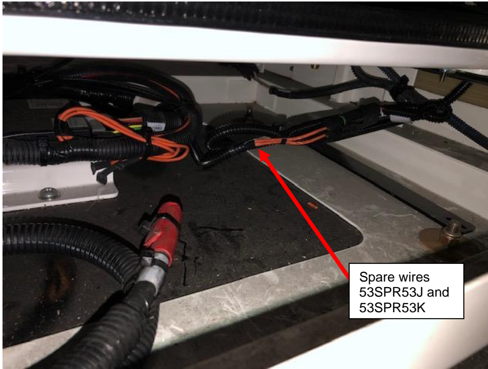
Figure 11: Exterior, street side work area access, inside bottom of SDS cabinet
