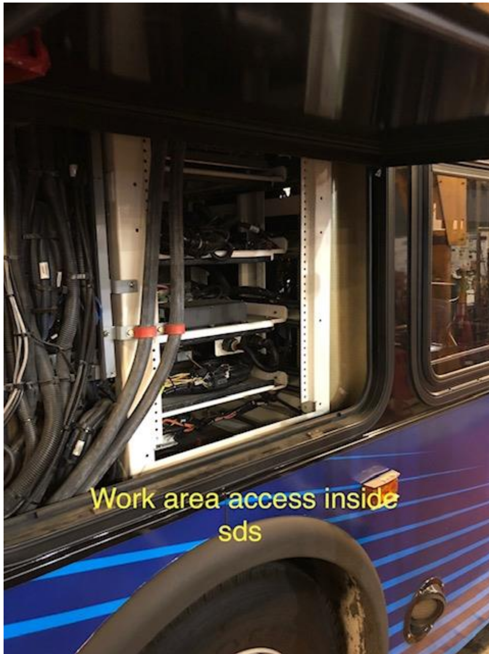
Figure 2: Exterior street side work area access inside SDS cabinet
