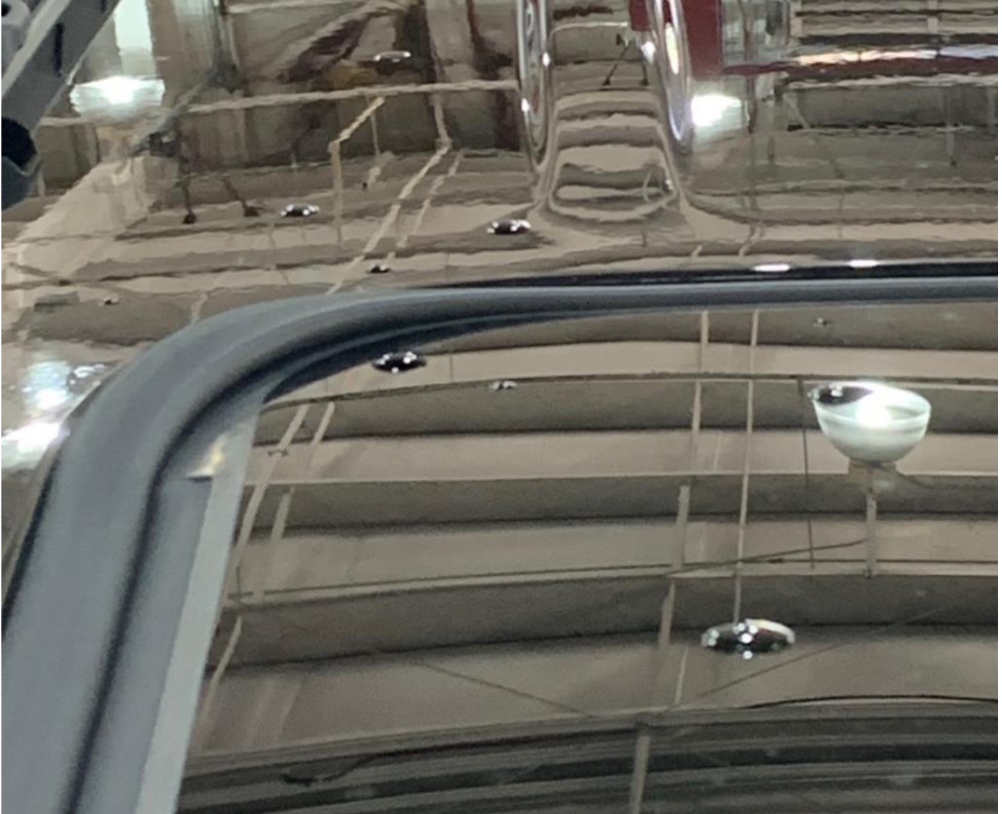
Fig 2 Example of sunroof exterior seal lifted
