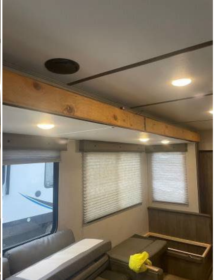
HEADER AFTER REMEDY
