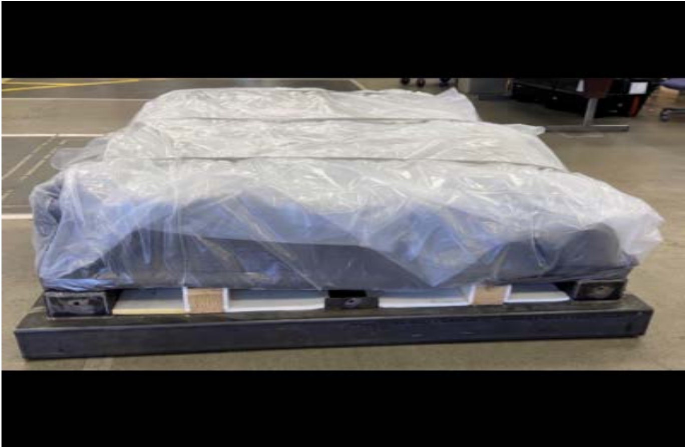
28. Completed wrapped battery.
