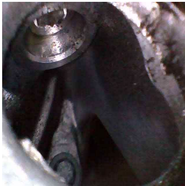
Figure 1. Missing sealing cap viewed with a pocket mirror.
