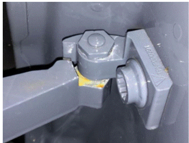
Figure 1. Visible signs of corrosion on the door hinge.
