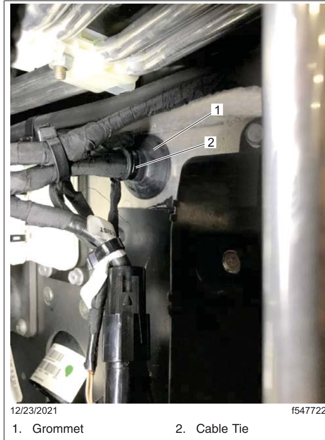
Fig. 12, Firewall Grommet and Cable Tie
