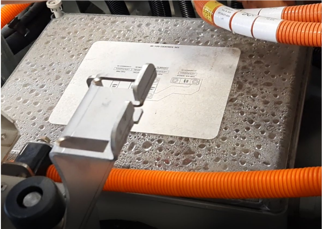
Figure 3: Fuse Box Condensation
