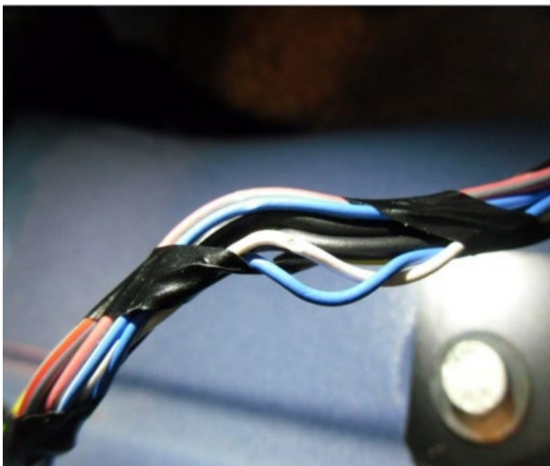
Figure 3: Example of a possible problem on the I-CAN line (white wire and blue wire) for the HVACR control unit).
