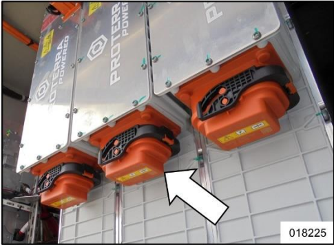
Figure 24: Location of manual service disconnect (MSD) (one on each of the nine batteries)
