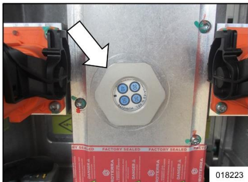
Figure 9: Desiccant saturation window unit shows an uncontaminated pack
