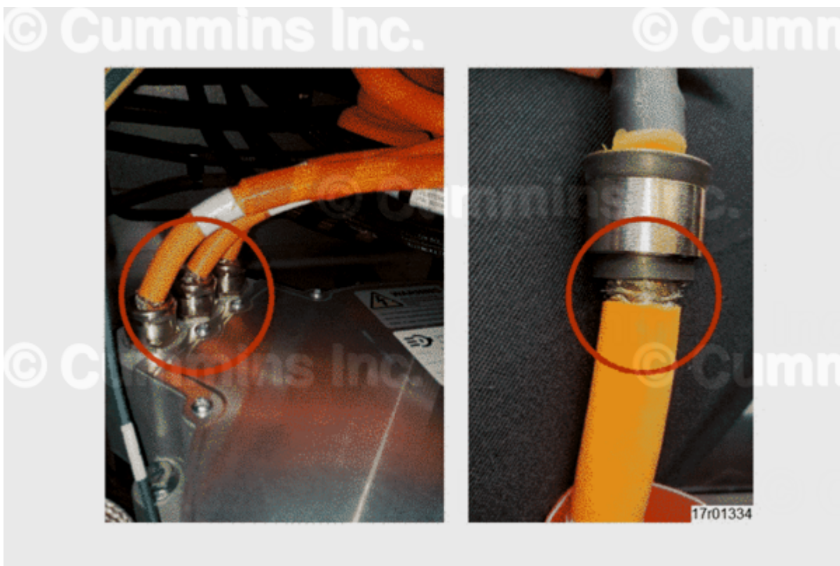
Figure 1, Example of Exposed High Voltage Cable Shielding.
