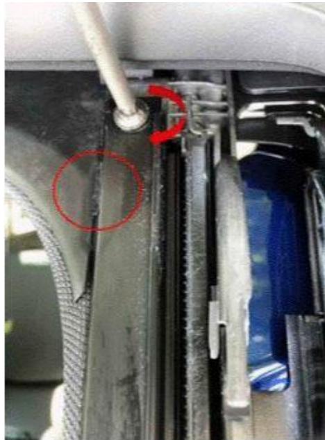
Figure 14. Tightening of the screw with the felt strip material isolating the guide rail and the frame.
