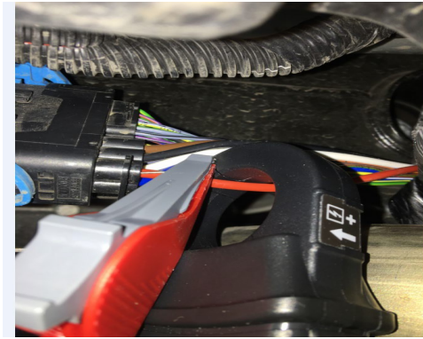
Figure 10: Power supply wiring to the air suspension compressor.
