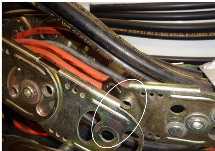
Figure 13 – Bent and Detached Links
