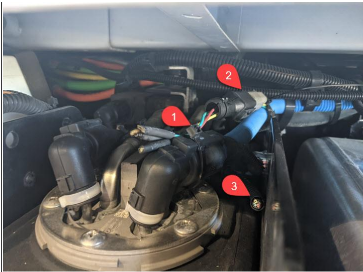
Figure 8: QLS Pigtail Installed
