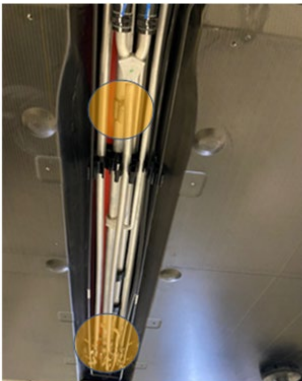
HVAC pipes along centre of vehicle tunnel
