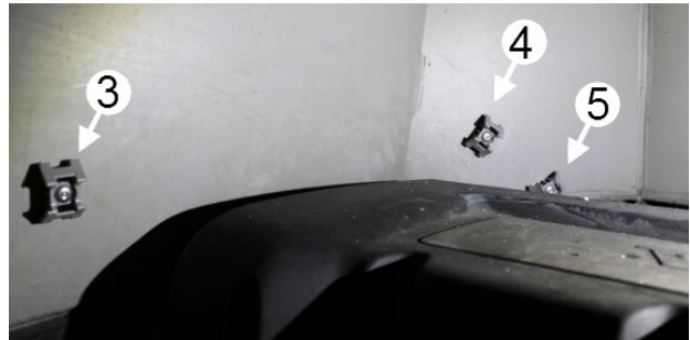
FIGURE 115: TIE MOUNT 3 & 4 SHALL NOT BE PLACED BETWEEN THE BULKHEAD AND THE VALVE COVER.
