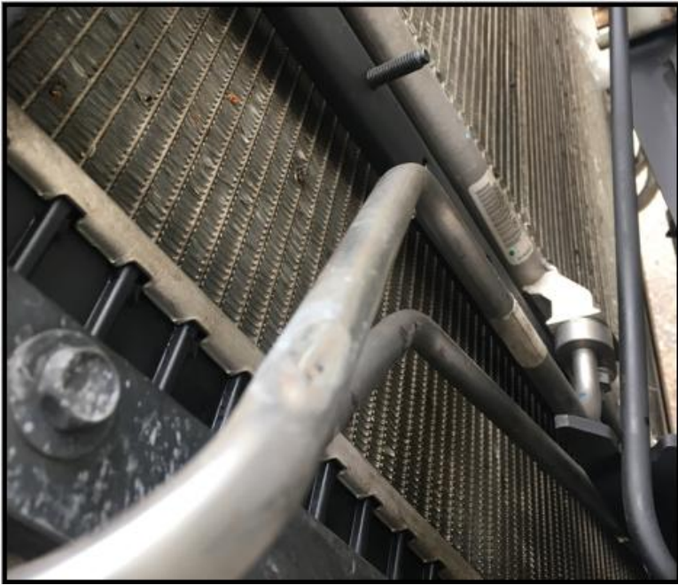
Figure #2: Upper hose has contacted hood assembly.
