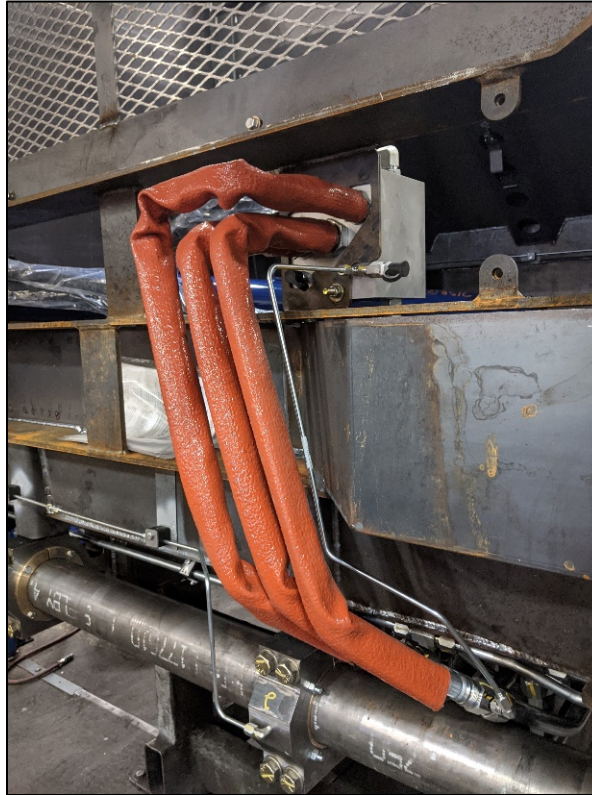
Figure 2. Front Head Tubes with Thermal Resistant Sleeves Installed (1/4" Tube Sleeve Not Yet Installed)
