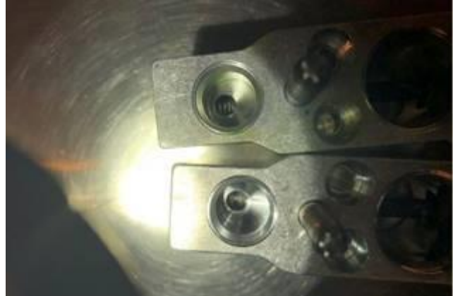
Figure 4. Leak at expansion valve connection evidenced by residue from the contrast agent.
