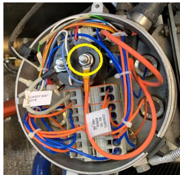
Figure 19: High Voltage Positive Auxiliary Heater Connection
