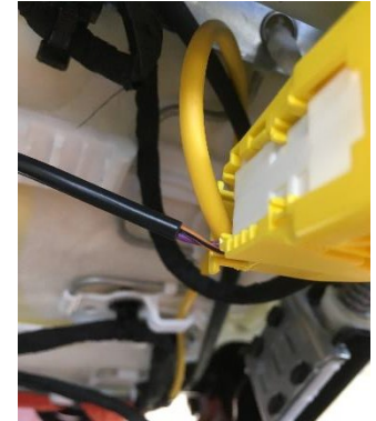
5.4 Condition without cable tie
