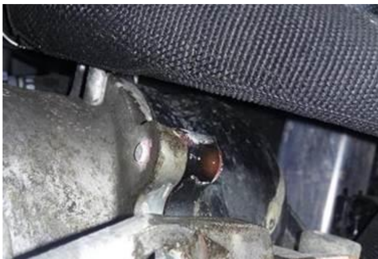
Figure 5. Coolant marks on coolant connector union.
