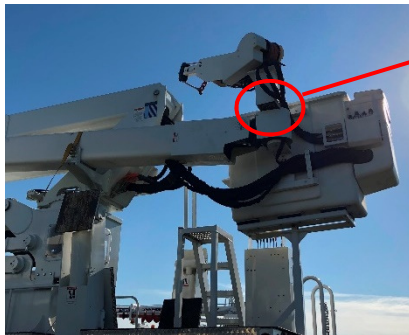
Figure 15. Jib storage limited to eliminate over rear position, this update may not apply
