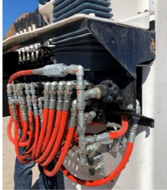
Figure 9. Upper control valve extra return line and vent not added, this update applies
