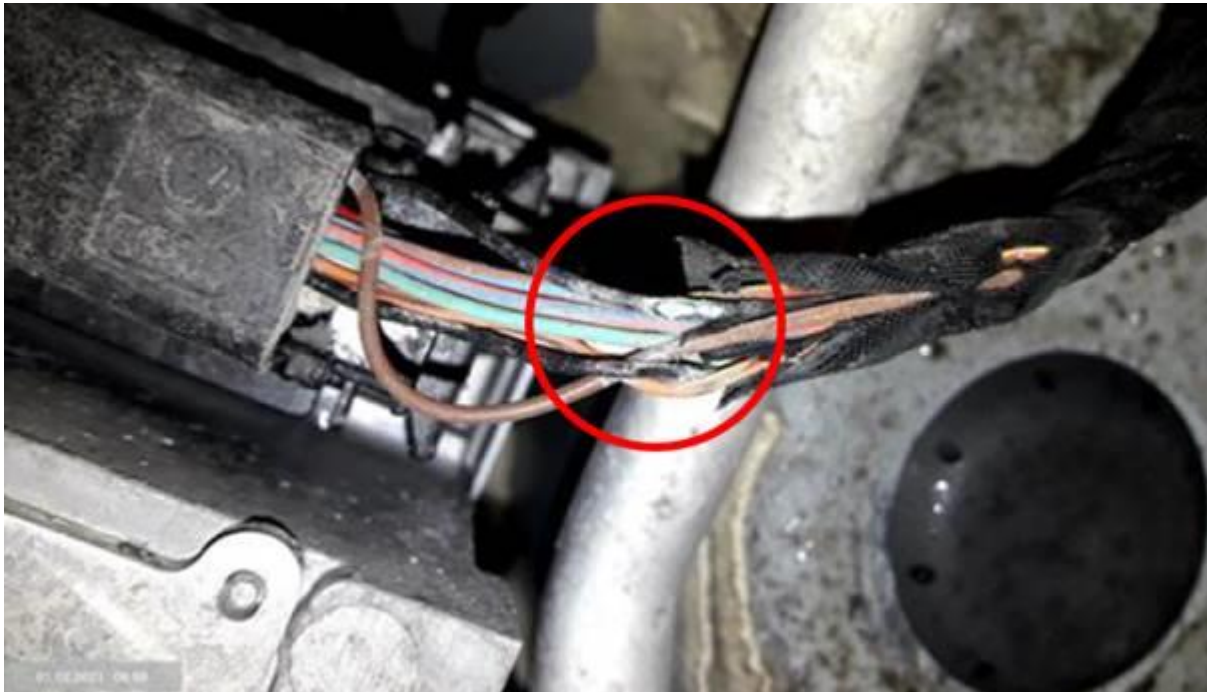
Figure 1. Chafed 12volt harness section.
