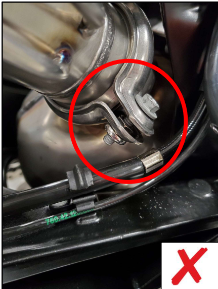
Fig.1 - Incorrectly mounted clamp
