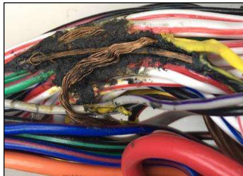
Fig. 6 - Severe Damage (follow code 02)
