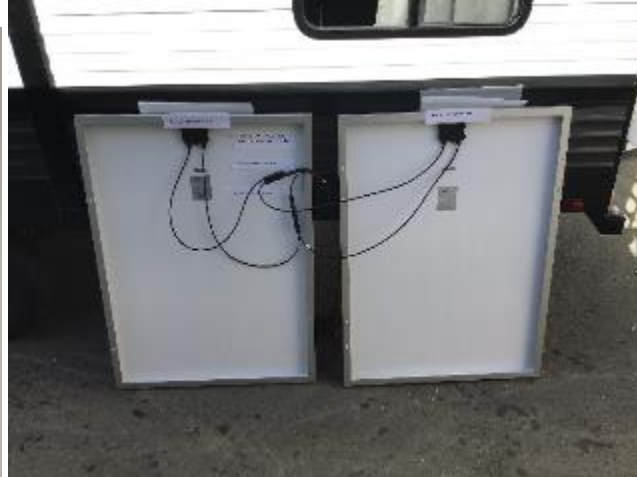
FIG - 8 Primary & Secondary Solar Panels Connected
