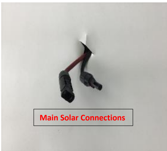
FIG - 3 Main Harness at Roof from Solar Controller
