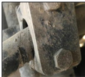
Figure 5. INCORRECT Use of Tube Clamps for Hoses
