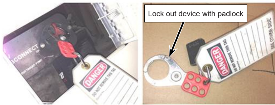
Figure 3 - Battery Disconnect Switch Locked Out in OFF Position
