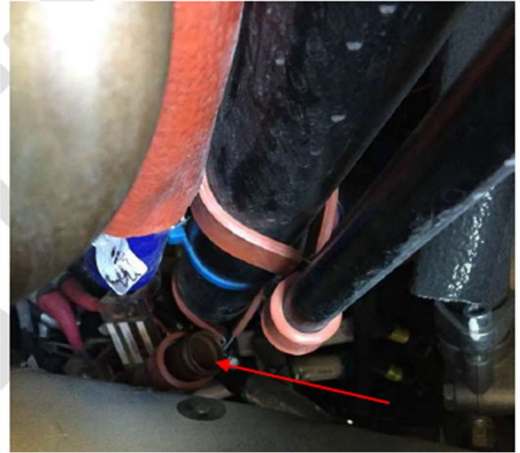
Outlet side of heater
