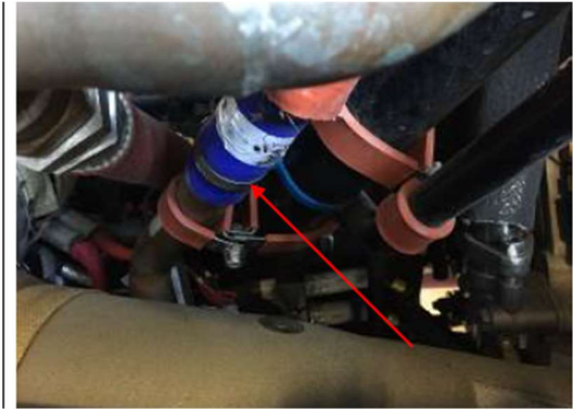
Outlet side of heater
