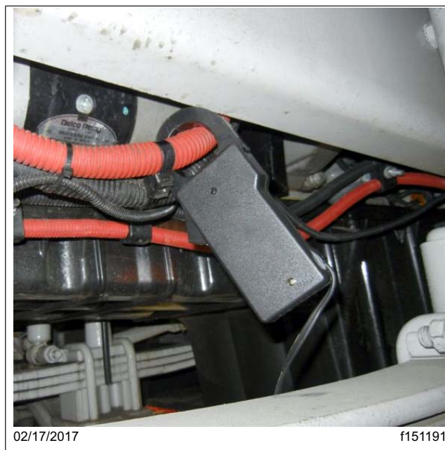
Fig. 9, Measure the crank amperage with an amp clamp on the positive starter cable during crank.
